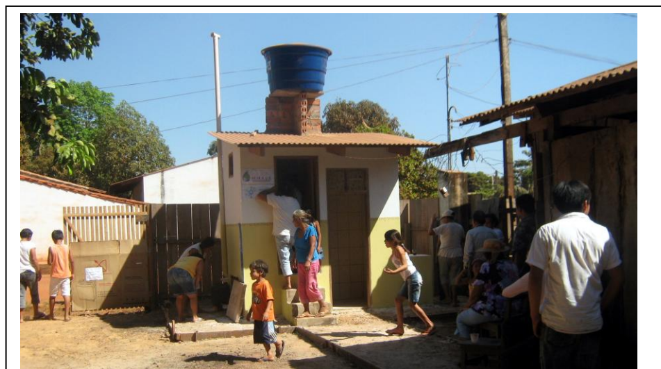
DSSN is building ecosan toilet modules in 400 households in the Bolivian Amazon
