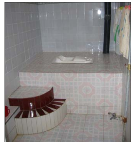
Figure 1: Urine-diverting double-vault dry toilet built indoors (Guangxi Province, China)
