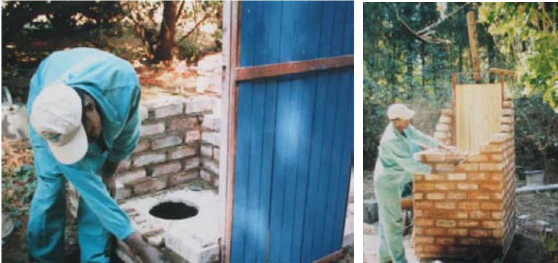
The steel frame is mounted again on the slab and the same bricks are used to rebuild the structure.
