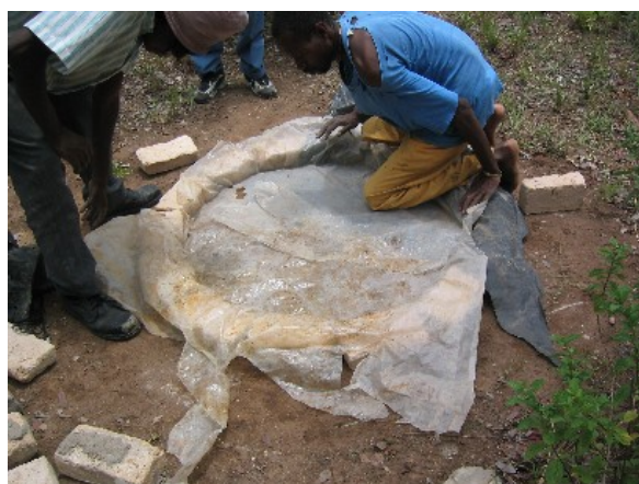
The squat hole is made by placing a shaped plastic bucket or shaped bricks in the slab mould.
