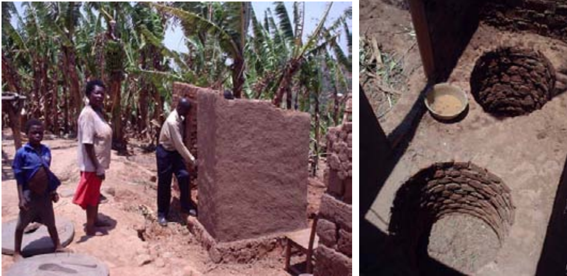
On the left a permanent brick Fossa alterna structure is built around two brick lined pits in Thyolo, Malawi (COMWASH Project). The brick lined pits are shown on the right.
