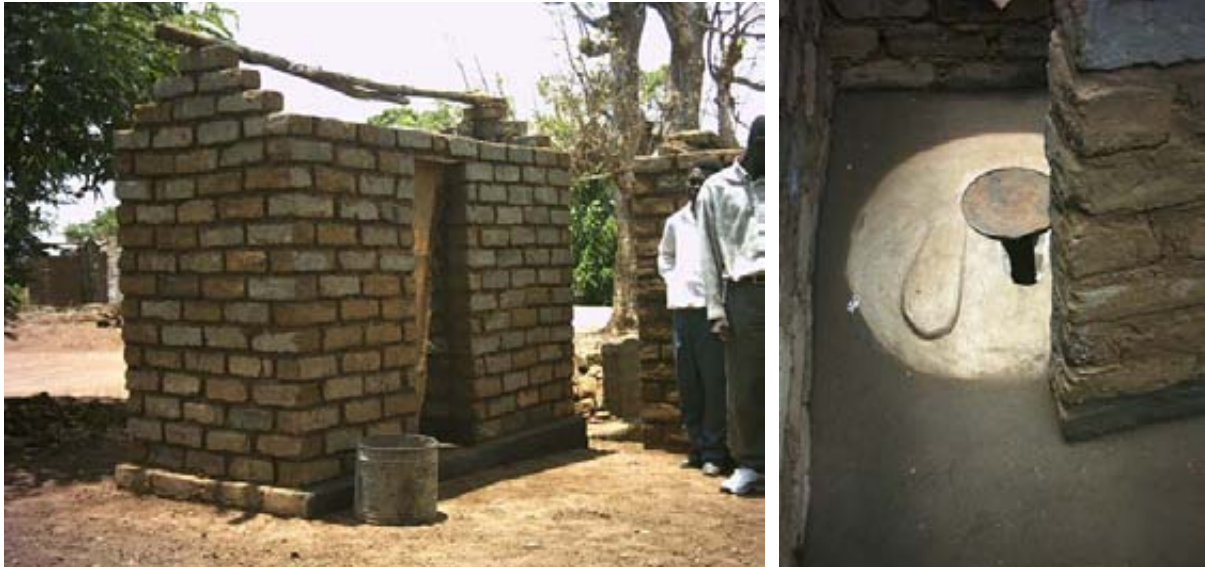
Very neat Fossa alterna constructed in peri urban settlement near Lilongwe. The roof has still to be added. On the right a view of the interior with round domed slab.
