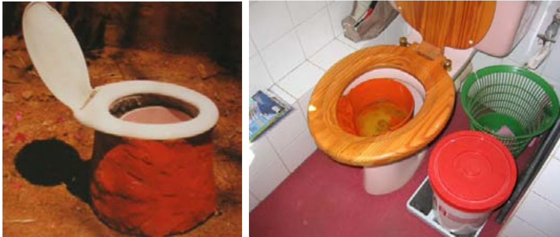
On the left a 10 litre bucket is placed beneath a pedestal which helps women to collect urine. On the right a urine collector shaped from a plastic bucket is used to collect urine from a standard flush toilet.
