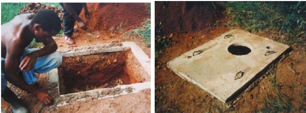
Adding a layer of weak cement mortar for the slab to rest on. This helps the slab to rest on the ring beam without strain. Also if a vent pipe is used, the pit should be air tight, thus allowing the suction of the pipe to draw air down the squat hole or pedestal. This leads to odourless conditions in the toilet. On the right a slab is mounted over the ring beam. This slab has a larger hole intended for a pedestal cast in it.
