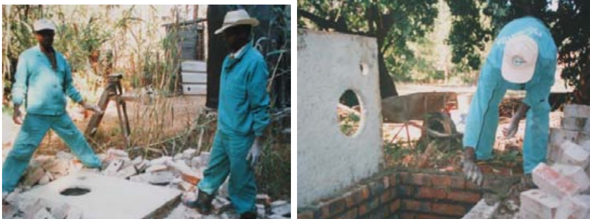
All the brickwork has been taken apart. The bricks are cleaned up. This is easy because the mortar is weak (20:1 sand and cement). On the right the same slab, having been removed from the original pit, is relocated on the second pit and mounted over a bed of weak cement mortar.
