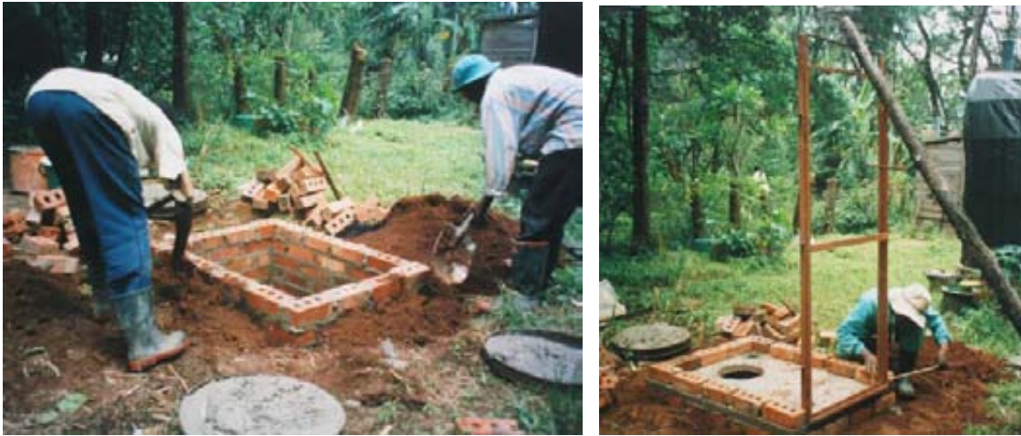
One of the two pits is dug and lined with cement mortared fired bricks. The steel frame (with door frame) is erected at the “door” end of the slab and the brick walls are built. “Sprags” of steel welded to the frame link the steel component with the brick and mortar work.
