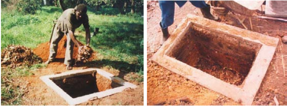
Adding dry leaves to the base of a pit helps the composting process. A full sack full or even two sacks full works well. The pit is ready – ring beam in place and leaves at bottom.
