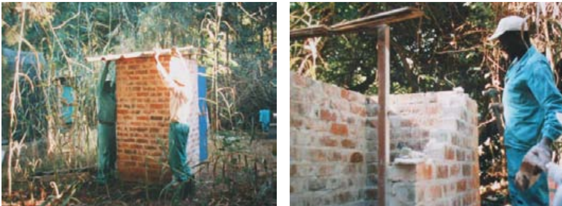
The roof is fitted after completion of the brickwork and door fitting. An asbestos pipe will also be fitted. Photo on right shows first stage of dismantling. The pipe, pedestal and roof have been removed. Now the brickwork is taken apart.
