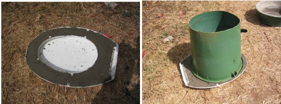
A strong mix of concrete using 3 parts river sand and 1 part cement is mixed and added to the toilet seat as shown. This will add strength to the seat and form a bond between the seat and side walls of the pedestal. The bucket is now fitted centrally over the toilet seat as shown.
