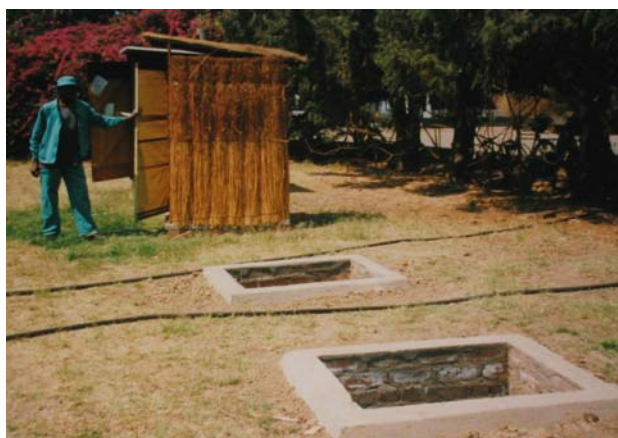
This Fossa alterna is actually used in a heavy duty communal setting. Three pits have been built to cope with the use.
