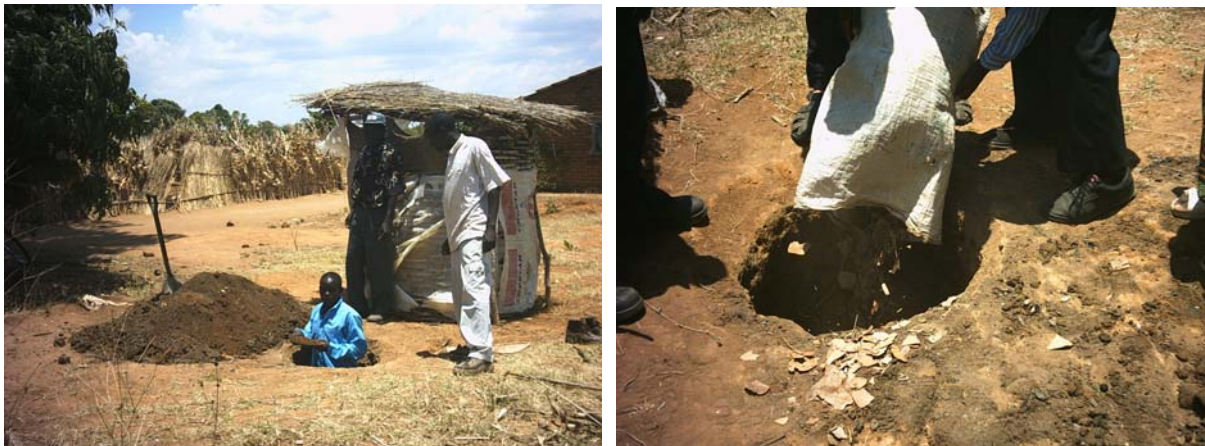
Excavation of Fossa alterna pit in Embangweni. In this case the structure is a simple bamboo portable unit which is moved from one pit the other. The ground is very firm in this locality and no ring beam or pit lining was used. The pit took less than 30 minutes to excavate and the entire operation of excavating and moving the slab and structure to the newly excavated pit took less than one hour. On the right dried leaves are being placed down the new pit. These help to compost the excreta like the soil which is added.
