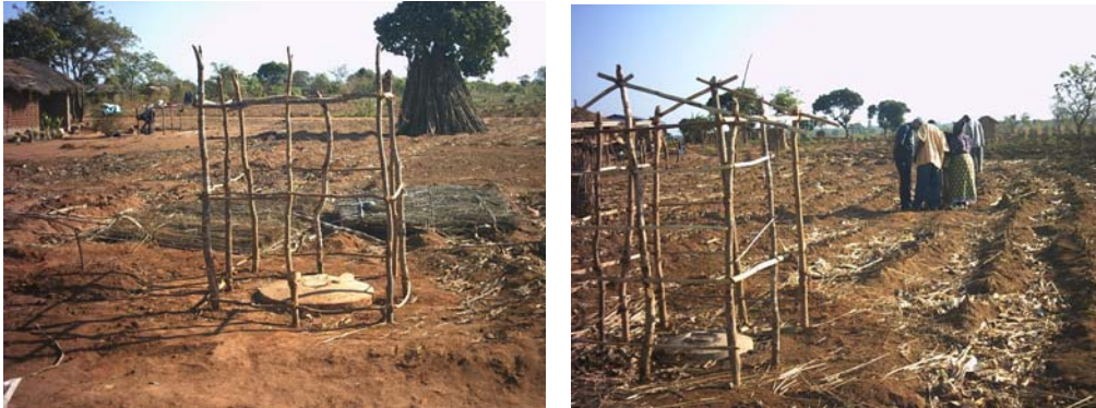
These Arborloos built in Embanweni, Malawi, where the soil is firm, do not have any form of pit protection. The 0.8m diameter concrete slab is laid directly over a 0.6m diameter hole and the simple superstructure built on top. The pits are dug about 1.0m deep.
