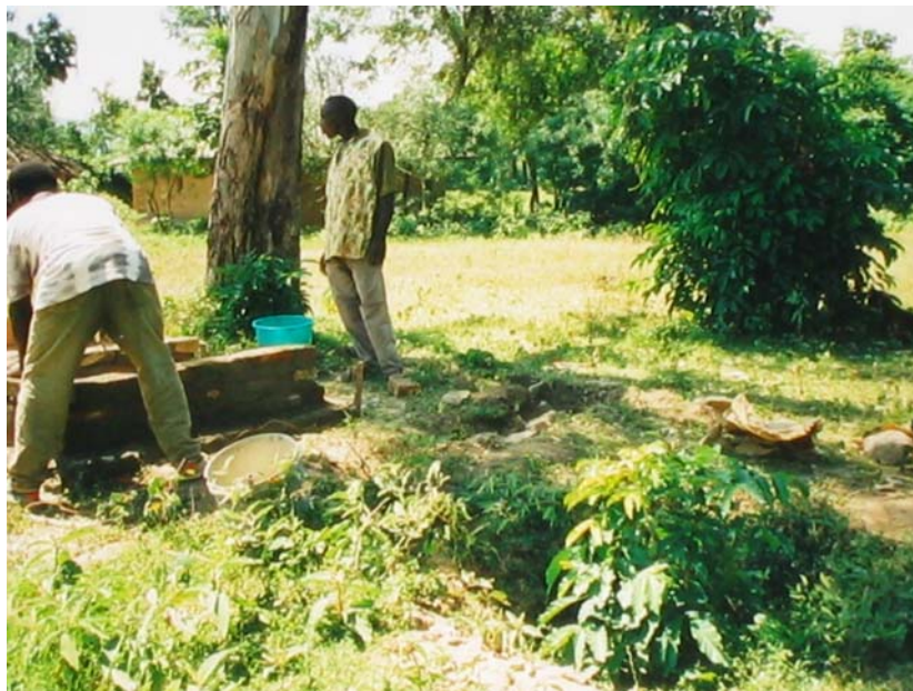
A new latrine is being built to the left. On the right is the depression left from an old latrine pit. Close inspection reveals that an indigenous tree is starting to grow there. Photo a Kusa Village, Kenya.
