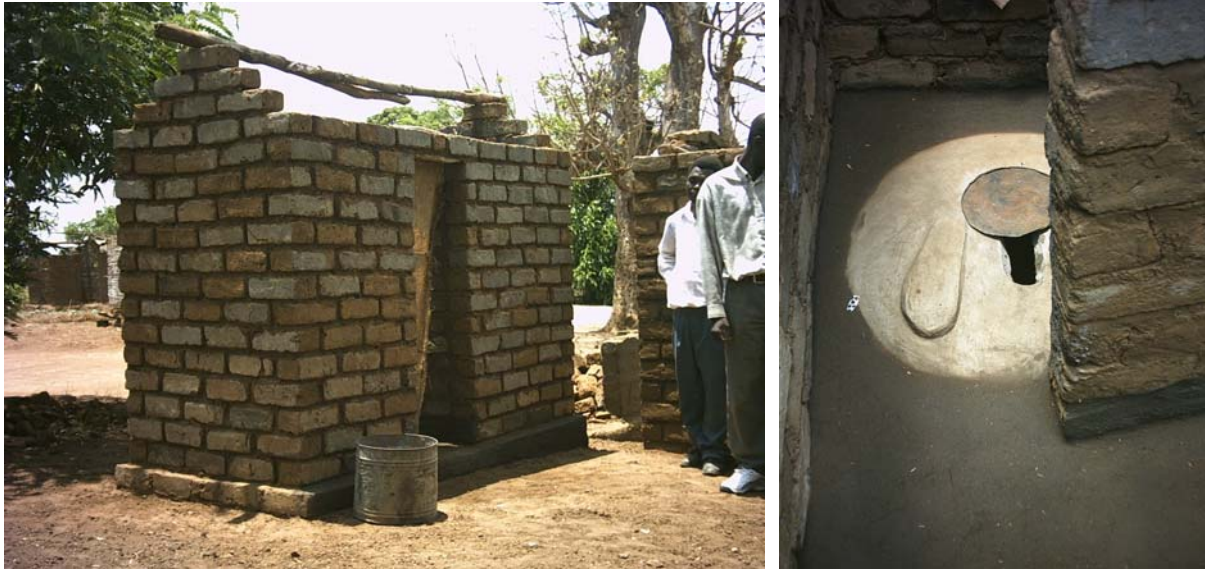
Very neat Fossa alterna constructed in peri urban settlement near Lilongwe. The roof has still to be added. On the right a view of the interior with round domed slab.
